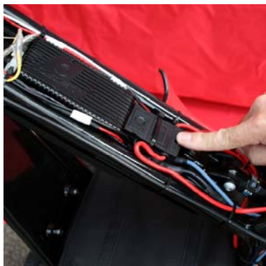
Controller and fuse.
